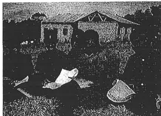
Figure 14-28 The NGO World Vision is helping the village of Kasanga, Uganda, to build this new school. When the school is completed, students will be able to meet in classrooms instead of under trees.
