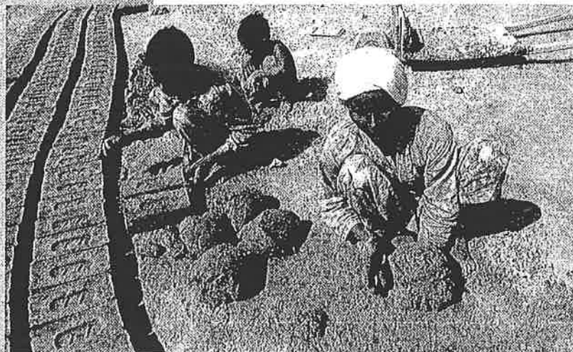
Figure 14-21 Young girls and boys work under scorching sun to construct this road in Batapur village, Pakistan.
